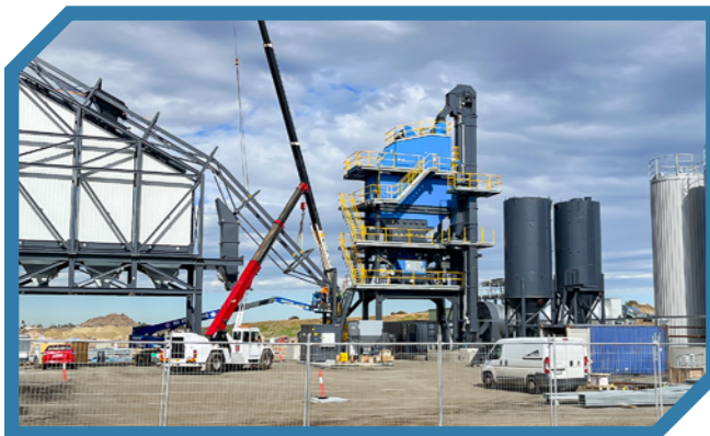
Hanson, Epping VIC, ashfall plant.
