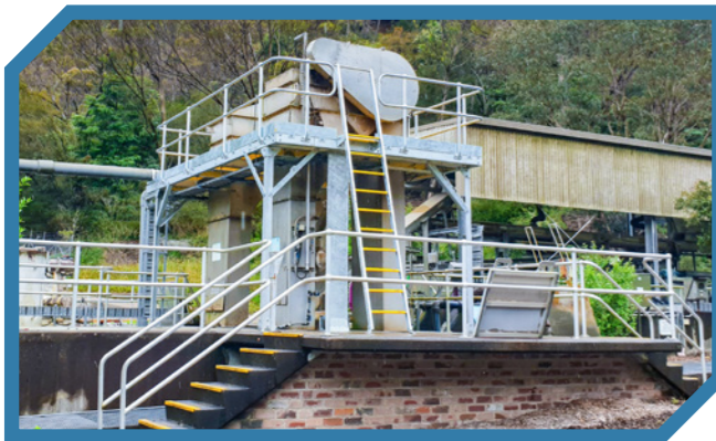
Sydney Water Hornsby Heights maintenance platform.
